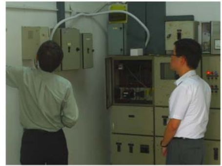
Professor Henry Chung inspected the installation in switch room.
